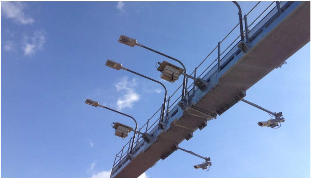
Figure 53 – SICK LIDARS on a SICE gantry.
